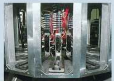
Interior of actuator units
